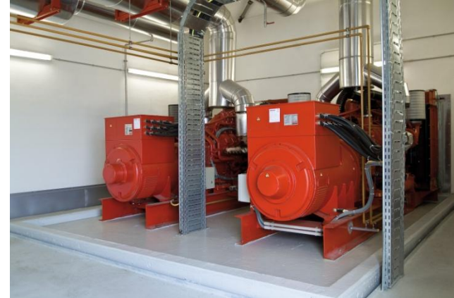
Emergency diesel generator
